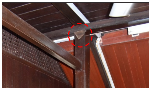
Figure 1. The remaining piece of cloth found on top of Tiang Seri
